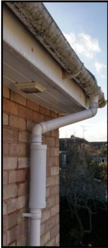
A) Chamber connected to downpipe
